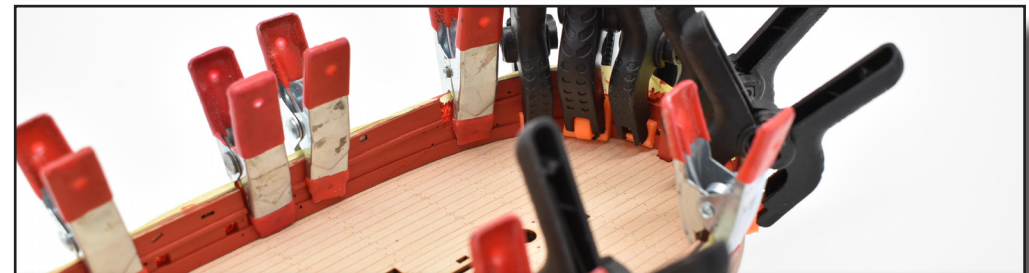
60. Again, using Plan Sheet 5 for placement, add the inner bulwark spirketting. For the prototype, PVA wood glue was used, and the parts clamped in place until the glue had cured, as shown.
