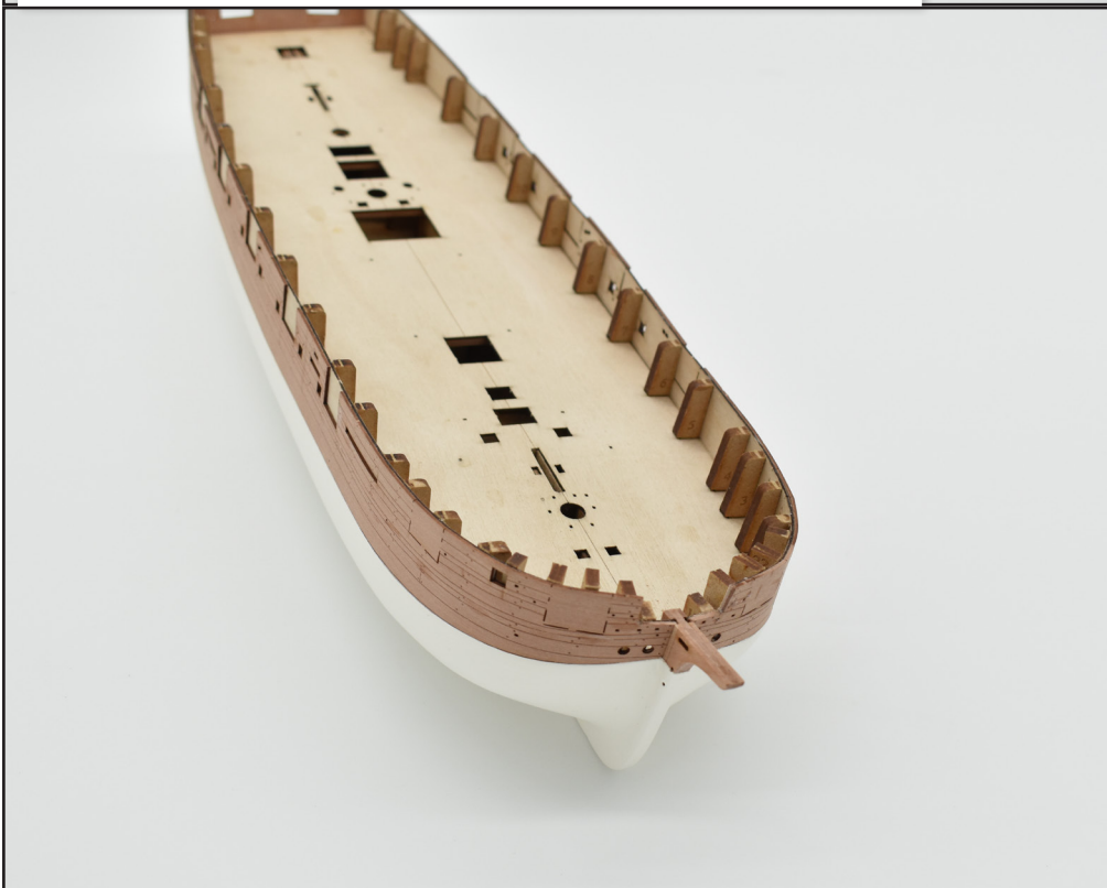
49. After 24 hours, remove the clamps. The bulwarks should now be firmly in place
